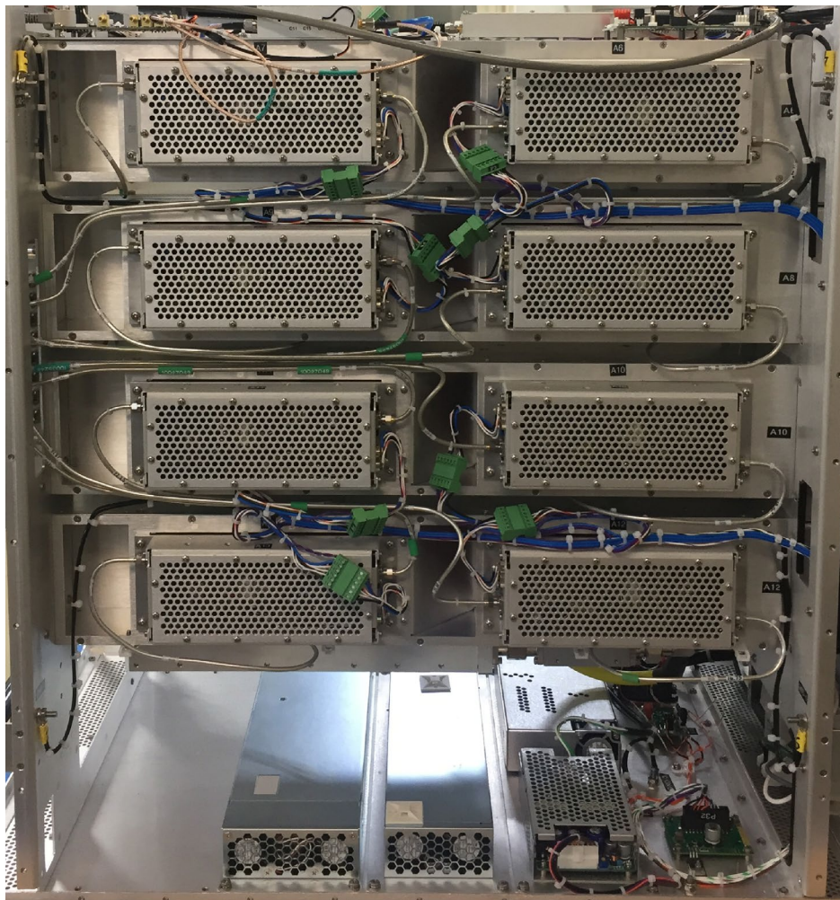
Figure 4-10. 1000W1000G, Right Side, Modules A6-A13.
